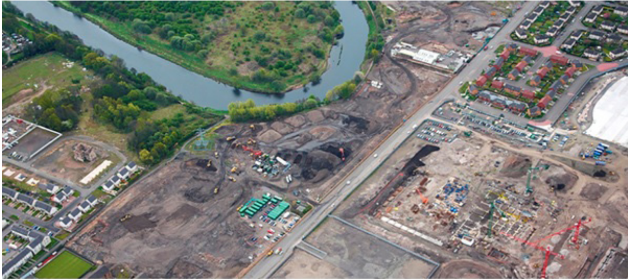
Figure 4.21: Aerial view of land preparation works for the Games Village (Courtesy of VHE Construction plc and GCC)
