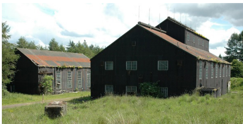
Figure 4.26: Outbuildings on the Former Royal Ordnance Site, June 2006 (Courtesy of Cass Associates)
